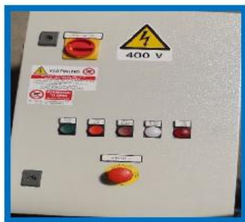
Electromechanical control panel
