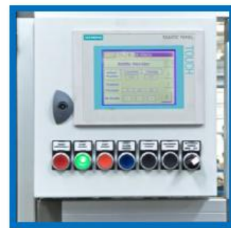
Divider control panel
